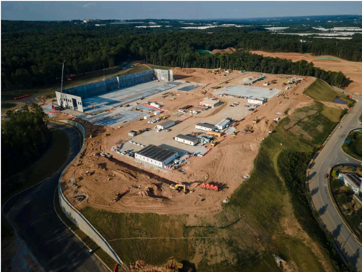
A construction site for a data center in Lithia Springs, Ga. The construction companies building huge data centers require IOS lots nearby to store their millions of dollars of tools, gear, tractors, trailers and other equipment. Dustin Chambers for The New York Times
